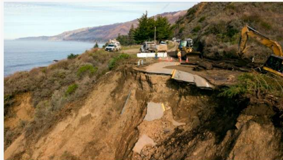
Construction crews work at the scene where a section of Highway 1 collapsed into the Pacific Ocean near Big Sur, California on Jan. 31, 2021. Credit: Josh Edelson/AFP via Getty Images.
